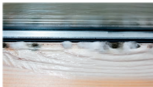
Mould is detrimental to health.
