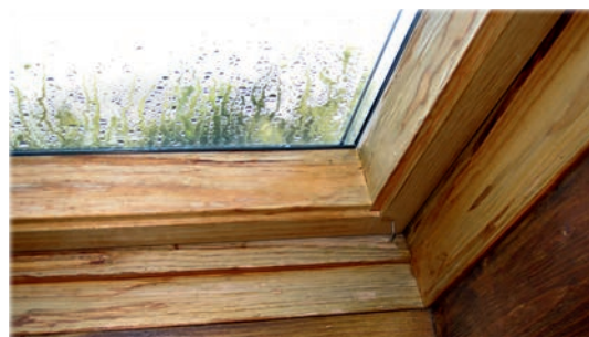
Condensation destroys windows.
